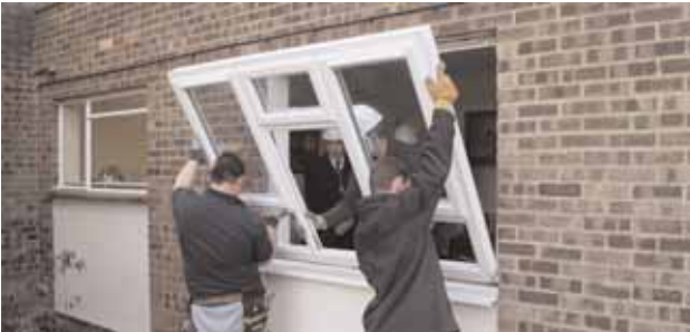
SECURING OF NEW PARTNERSHIP WITH CONNAUGHTS TO PROVIDE DAY TO DAY REPAIRS AND PH JONES FOR GAS SERVICING
